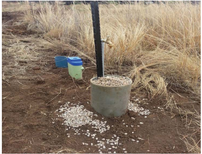
Tap and valve on the new water line
