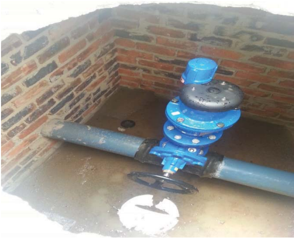
New Pipe water Network at Roodeplaas Nature Reserve
