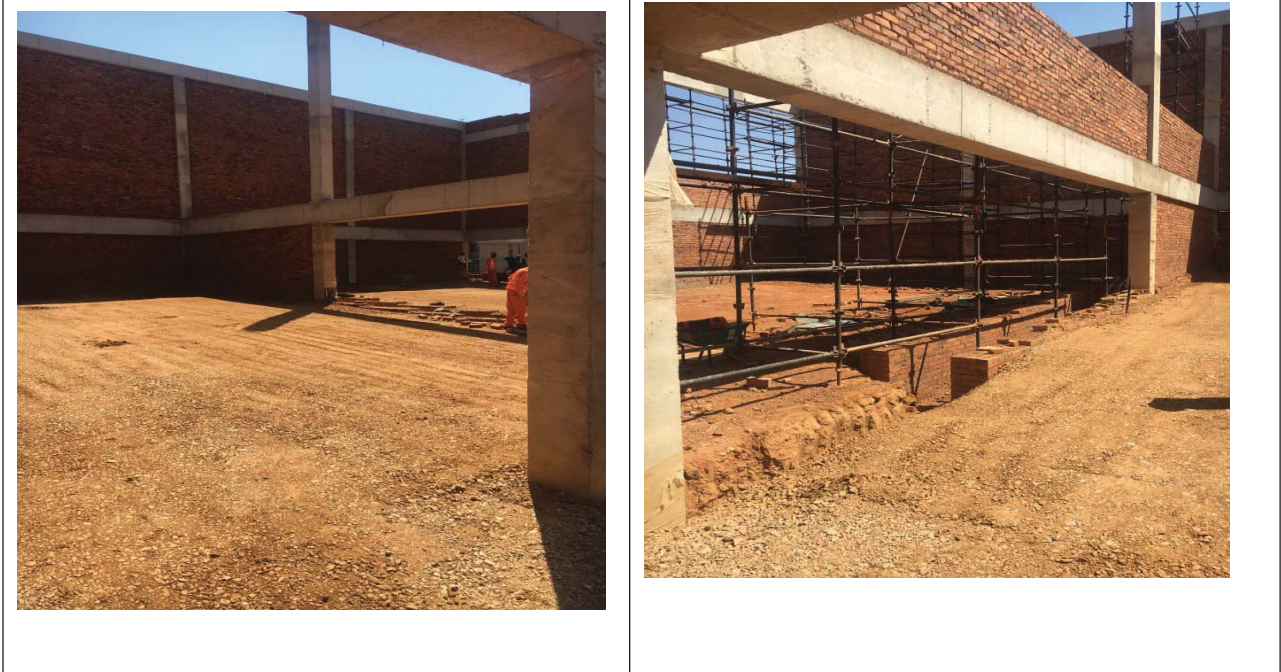
New Garankuwa Nurses College: Major concrete works have been completed Super structure at an advanced stage
