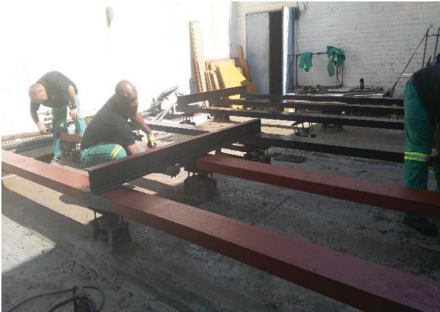
Bank of Lisbon building: Platform for the boilers & chillers
